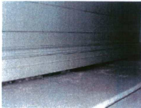
Gaps between floor and western wall Photo 1.11 June 2007
